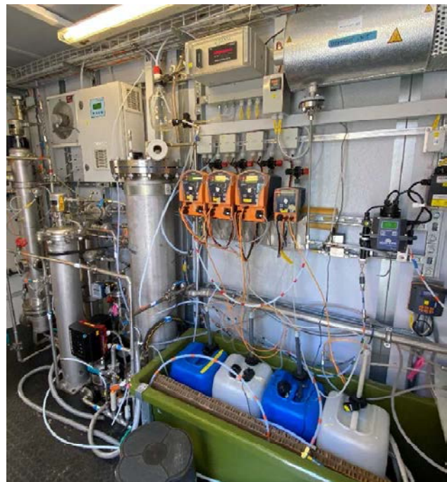
Figure 3-13. Ozone Pilot System
