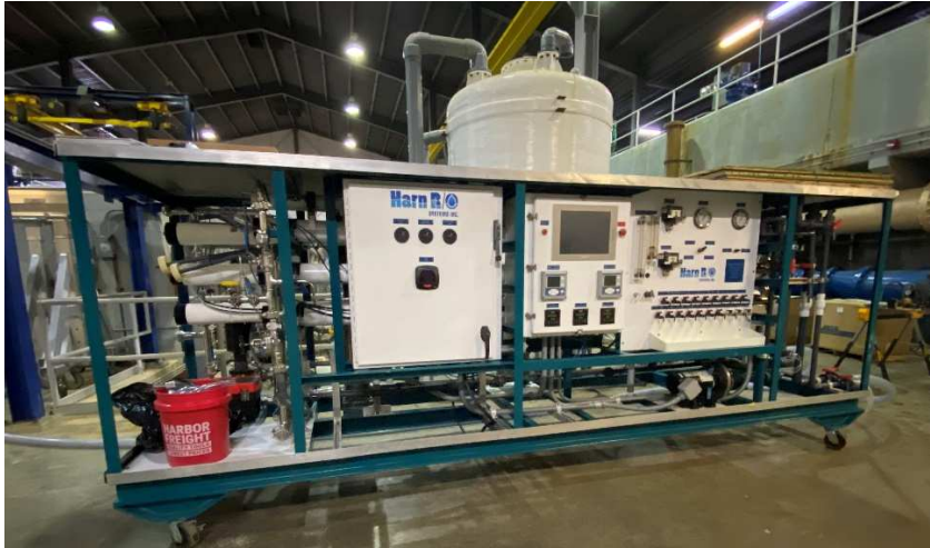
Figure 3-16. RO Membrane Pilot Unit
